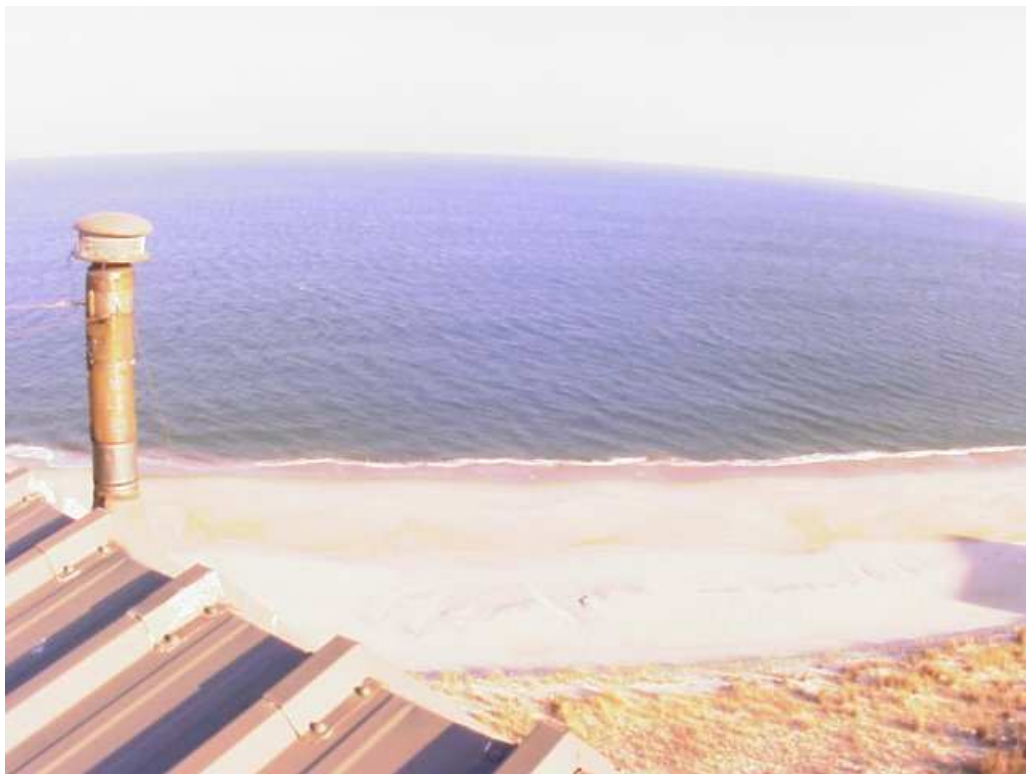
Figure A.1: The view from the Brandywine Building rooftop at the northeast apex. The exhaust stack obstruction is clearly visible, as is the sheet metal construction of the roof.
